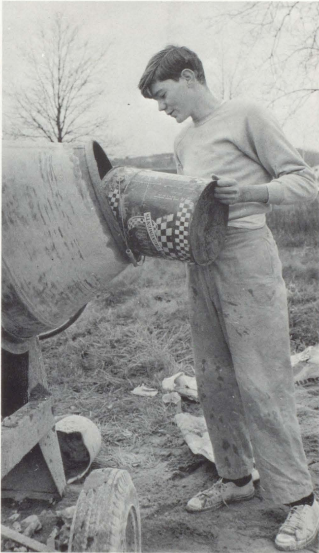
Mixing cement is a task that Senior Greg Weber must master in building and construction class.
