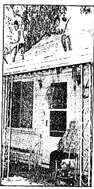
Homeowner Jayne Tremain eyes Corinne Atty, left, on roof and another student working.
