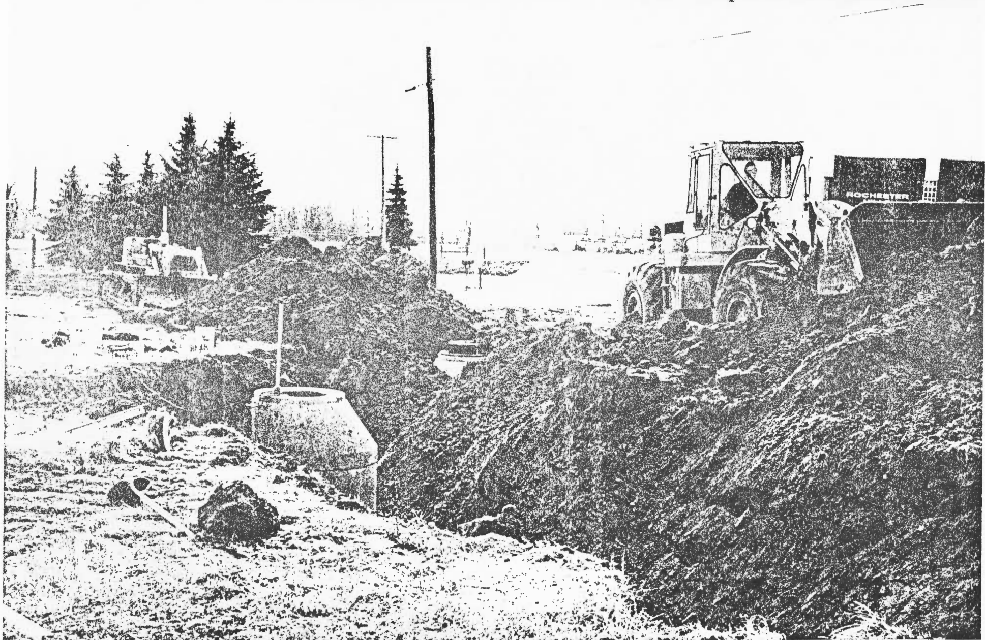
OAKLAND COUNTY DRAIN COMMISSIONER O.C.W.S. & S.D.S. Avon Twp. Ext. #2 Sewer Cont. #7 Contractor: Ric Man Location: M.H. 24A Photo No: 1 Date: 2/14/80 Photo by: Beth Singer
