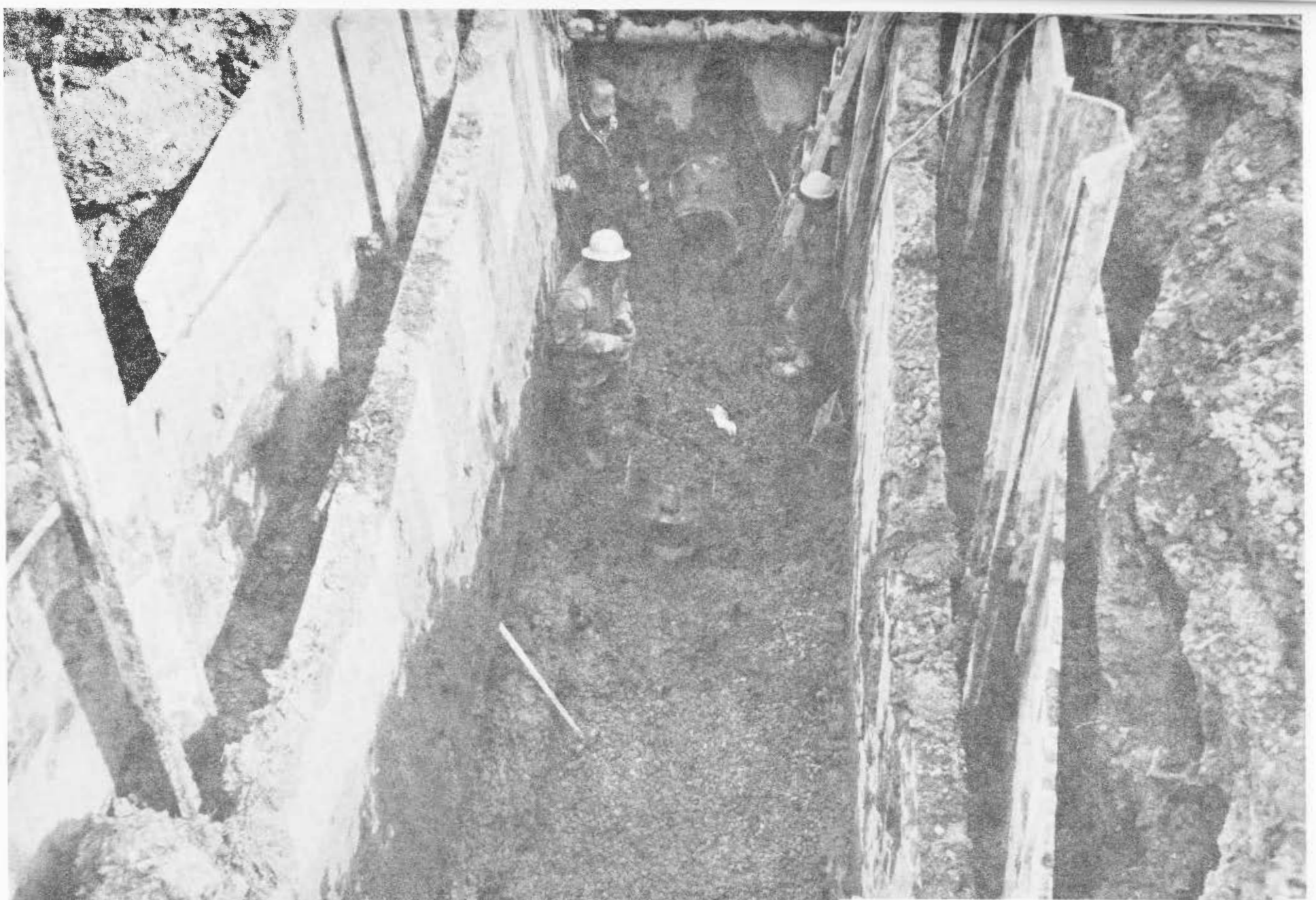
OAKLAND COUNTY DRAIN COMMISSIONER C.O.S.D.S. W. Bloomfield Ext. #2 Cont. #3 Contractor: Guy-Man Location: Under Bridge E. Rosedale Photo No: 4 Date: 3/4/80 Photo by: Beth Singer
