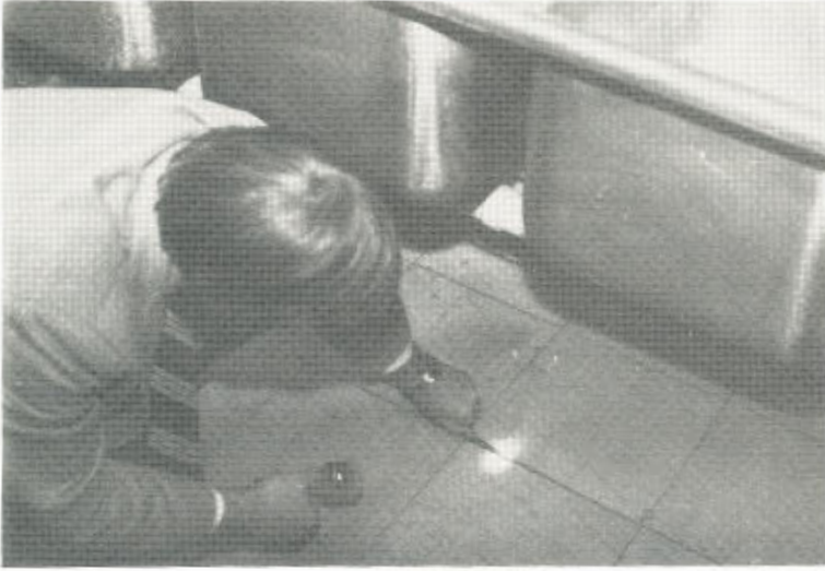
Floors in food service facilities must be clean and in good repair.
