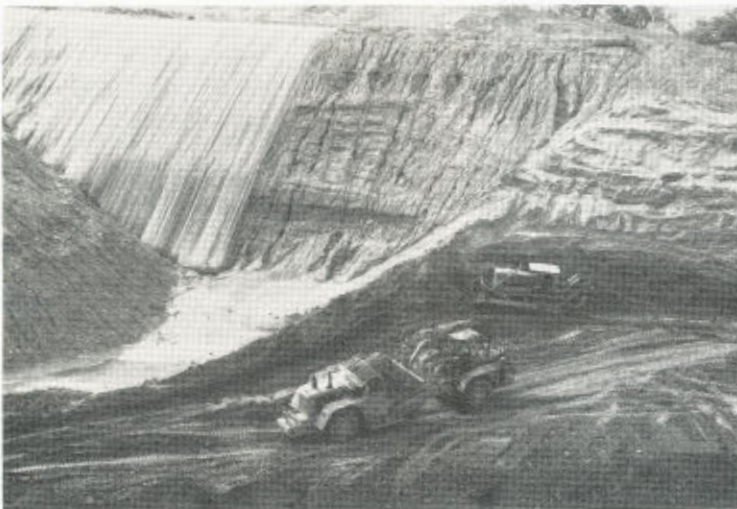
A plastic liner is needed at some sanitary landfills to protect the ground water from contamination.
