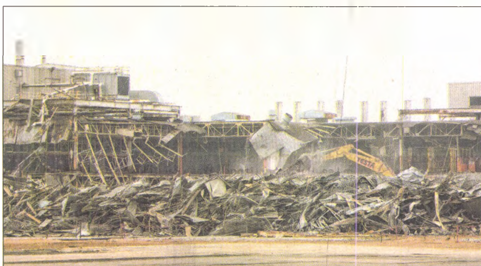
A backhoe from Testa Demolition continues work March 15, 2013, on tearing apart the Ford Wixom plant. The plant was about 50 percent demolished at that time, as work continued through the winter on taking down the 4.7 million-square-foot plant. Trident Barrow Management purchased the rights to develop three-quarters of the property in the future.
