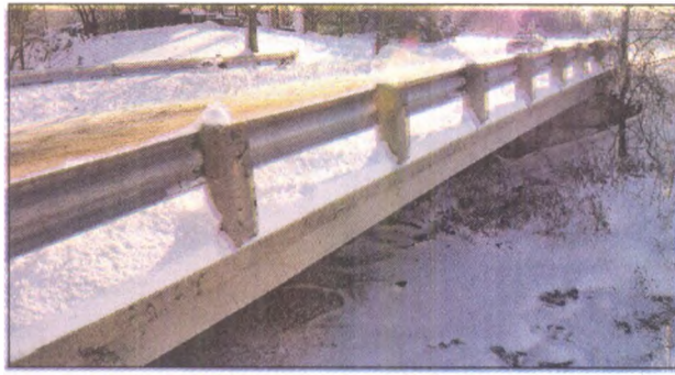
The city of Novi is planning on performing maintenance on a number of small bridges in the community, including this one on Willowbrook near Village Oaks Elementary. JOHN HEIDER | STAFF PHOTOGRAPHER
