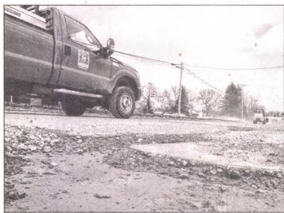
A Novi DPW pickup truck and Bobcat (far right) travel Feb. 24 down 11 Mile Road to help smooth out its winter-worn pavement. The road, west of Meadowbrook, already in tough shape from years of use, has been torn up from this year's severe weather.
