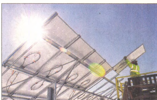
Chris Schear, an electrician for Ranck Electric, helps guide into place one of the 3,000 solar panels that are going up in Lyon Township along I-96 near Old Plank Road. Each panel should be able to generate, at peak wattage, about 700 watts of electricity. JOHN HEIDER | STAFF PHOTOGRAPHER
