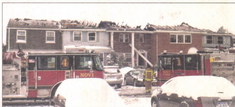
The Novi Fire Department responds to a blaze at Novi's Olde Orchard Condos. JOHN HEIDER | STAFF PHOTOGRAPHER
