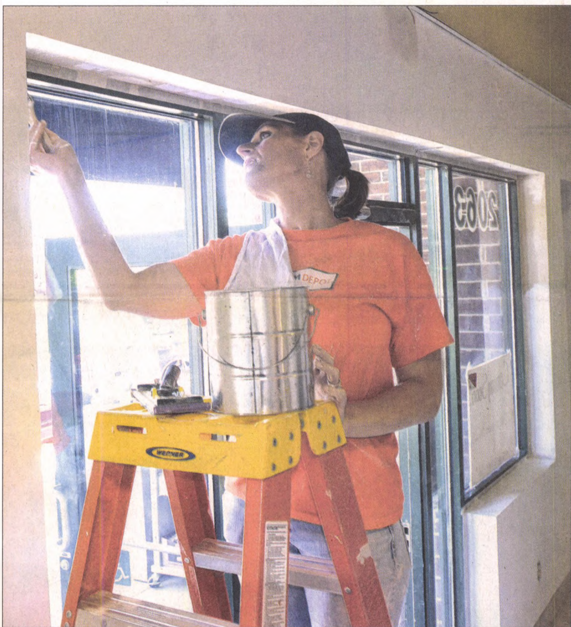
Amy Stump joins a group of Home Depot volunteers June 5 as they rehab the American Legion Constitution Post 224. JOHN HEIDER | STAFF PHOTOGRAPHER
