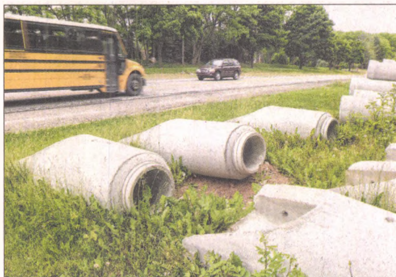
Drainage pipes are piled along the north side of Eight Mile east of Beck June 10 in anticipation of the start of a major effort to repair the stretch from Taft to Beck roads. JOHN HEIDER | STAFF PHOTOGRAPHER
