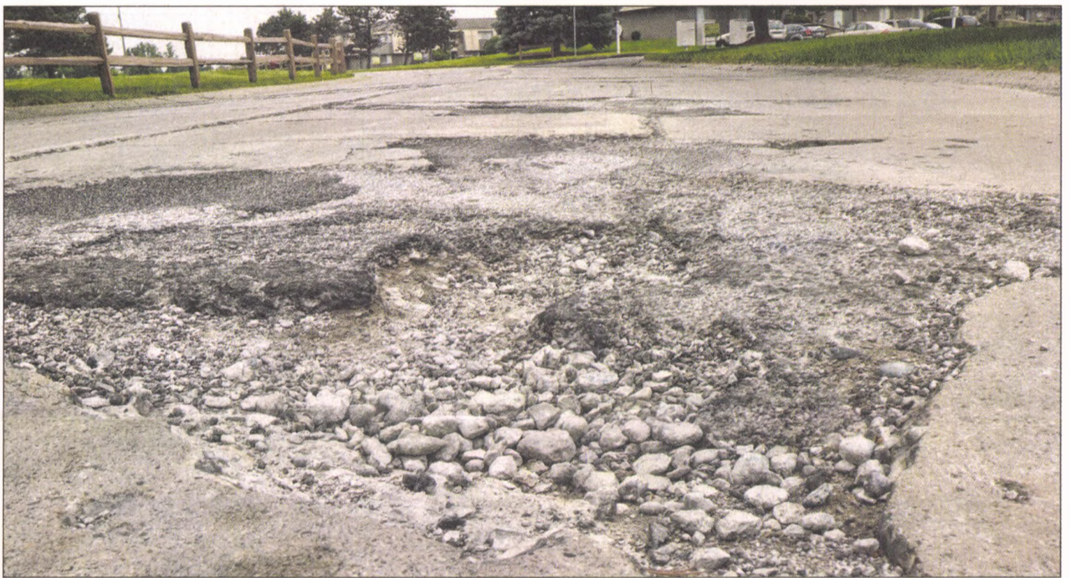
The city of Novi will be turning its attention to a number of side streets this summer for resurfacing, including this potholed section of Wedgewood off of Pontiac Trail. JOHN HEIDER | STAFF PHOTOGRAPHER
