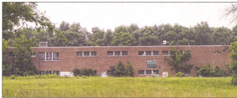
To combat trespassers and its slow collapse, the far western building of the former Northville Psychiatric Hospital on Seven Mile should be demolished soon. JOHN HEIDER | STAFF PHOTOGRAPHER
