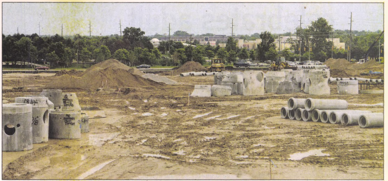
Work continues on the Northville Park Place development June 25 at Seven Mile and Haggerty. The first phase of the project is expected to open next spring. JOHN HEIDER | STAFF PHOTOGRAPHER
