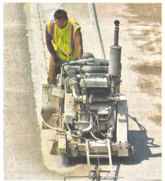
After the concrete sets, grooves are cut. When the road surface expands and contracts, the cracks should follow the grooves.
