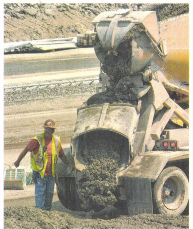
A constant stream of trucks dumps concrete that will become finished road surface, in a matter of minutes.
