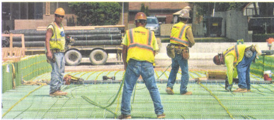
Reinforcing steel is laid before the concrete is poured for a new bridge surface.
