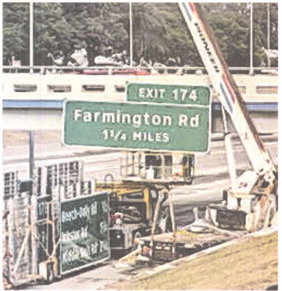
Michigan Department of Transportation officials say I-96 through Redford and Livonia could reopen by Sept. 30, several days ahead of schedule.
