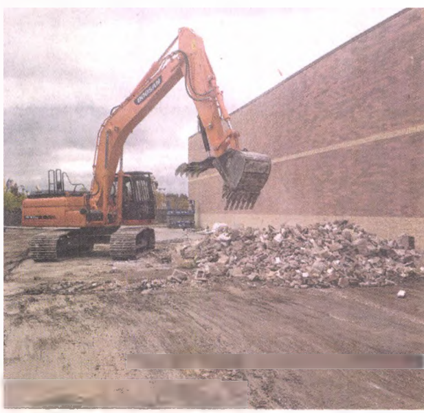
A crew from Detroit-based Blue Star Demolition begins the process of tearing down the former ABC Warehouse building on Ford Road to make room for expansion at IKEA.
