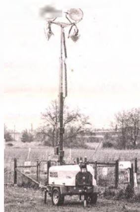
HAL GOULD | STAFF PHOTOGRAPHER The new lights have been installed at Lyon Oaks Dog Park.
