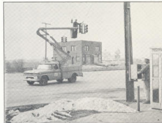
Routine check of traffic signal providing for safe operation.
