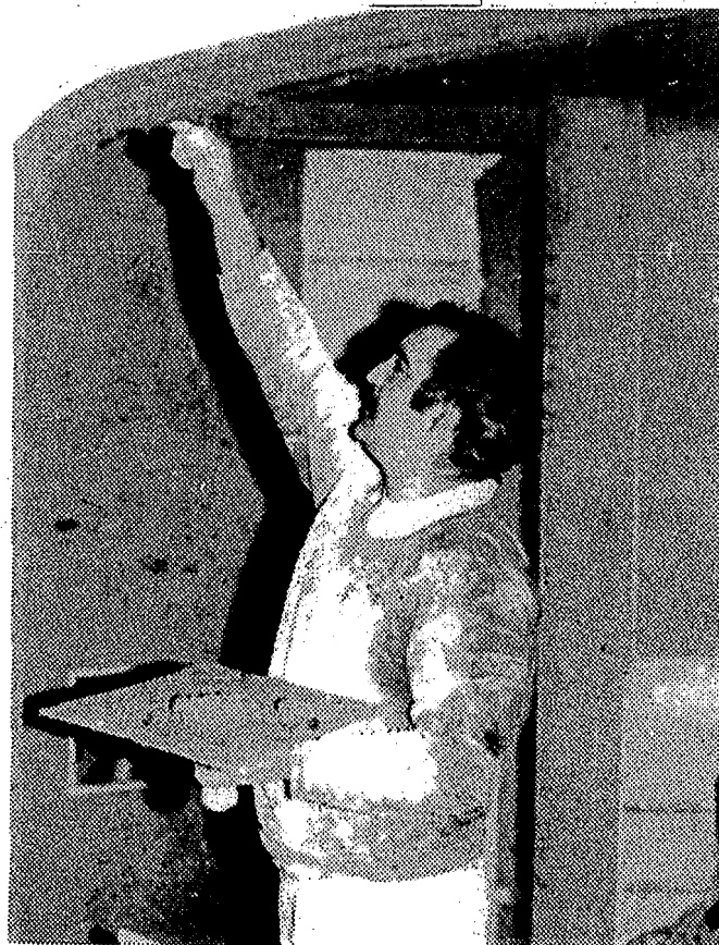
Every effort was made to find one of the finest plasterers in the area to duplicate the Mansion's Tudor arches.
