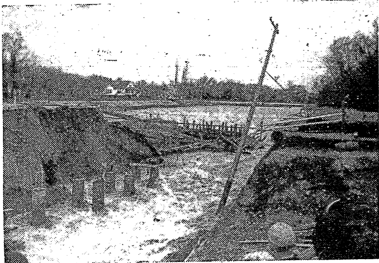
The above picture shows the flood of water just after the dam had burst. Note the four rows of concrete piers. The eighth pier was broken off and washed down into flooded area. Three minutes before this picture a man was out on the bank ten feet beyond the hanging electric light pole. Note also the mill pond in the background. News photo by Bud Yoh.
