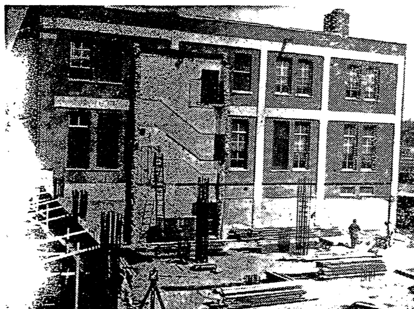
ABOUT CONSTRUCTION —$36,000,000 worth of buildings and equipment were added. This investment, all-time high for one year, would have been much greater but for continuing shortages of materials. Increasing demands for service and higher labor and material costs have raised the estimate for our 5-year post-war construction program to $220,000,000.
