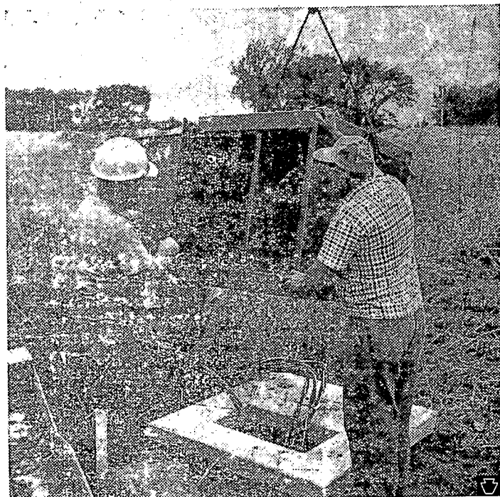
Weighing only 666 pounds and 28½ inches high, an Allis-Chalmers transformer installed in a Janesville, Wis., subdivision is easily maneuvered into place on its concrete pad. The subdivision is the first in the state with both electrical and telephone wires buried together in a common trench. The underground wiring system eliminates overhead poles and wires. Allis-Chalmers acted as general contractor for the entire project.
