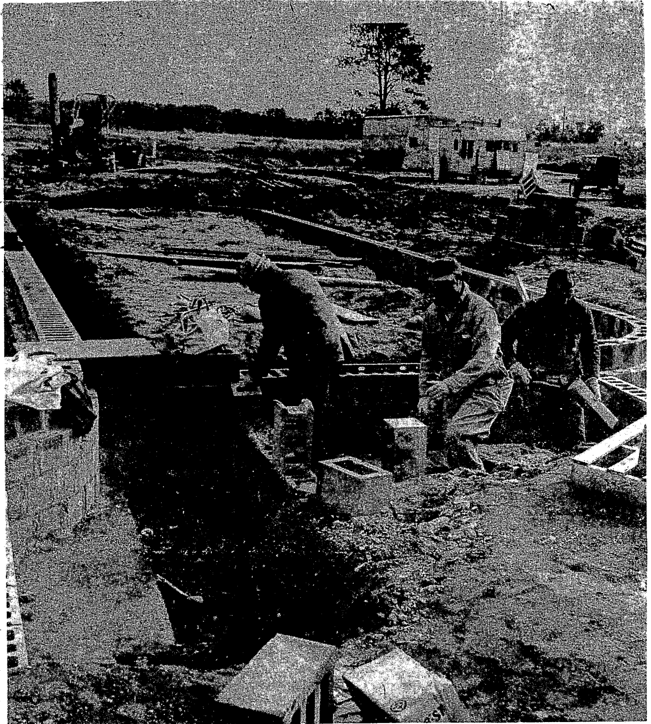
Construction was started on the Vocational Education Building which overlooks the intersection of Dixie Highway and I-75. Estimated maximum cost of the building is $1,207,900 which would include all work on the site and the 42,427-square-foot of building. Completion date is set for September, 1970 with the latest date, considering the possible delays caused by building trades complications, January, 1971. The building will accommodate approximately 550 students per day in 2 shifts. The curriculum will cover 11 occupational areas and will draw students from the school districts of Brandon, Clarkston, Holly, Our Lady of the Lakes, Waterford-Mott, Waterford-Kettering, and Waterford Township.
