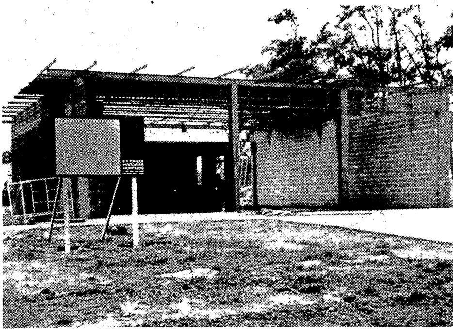
Construction on Independence Township Fire Station No. 3 at Maybee and Pine Knob Rds. is well under way.
