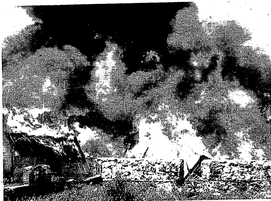
Independence Township firemen set fire to farm building on M-15 south of Oakhill Road recently as a part of the township's condemnation program for unfit habitations. The department kept watch as the barn (pictured above) went up in flames and smoke.
