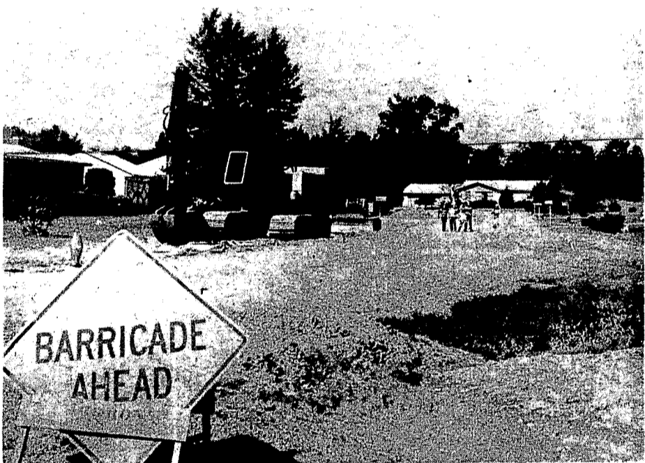
Residents of the Orchard, along Snowapple and Cramlane, have experienced firsthand the upheaval of sewer construction. Lawns have suffered, traffic has had to be detoured, and the rumble of giant machinery is a continuing item. By next year, sewage should be flowing to Detroit in the pipes now being laid.
