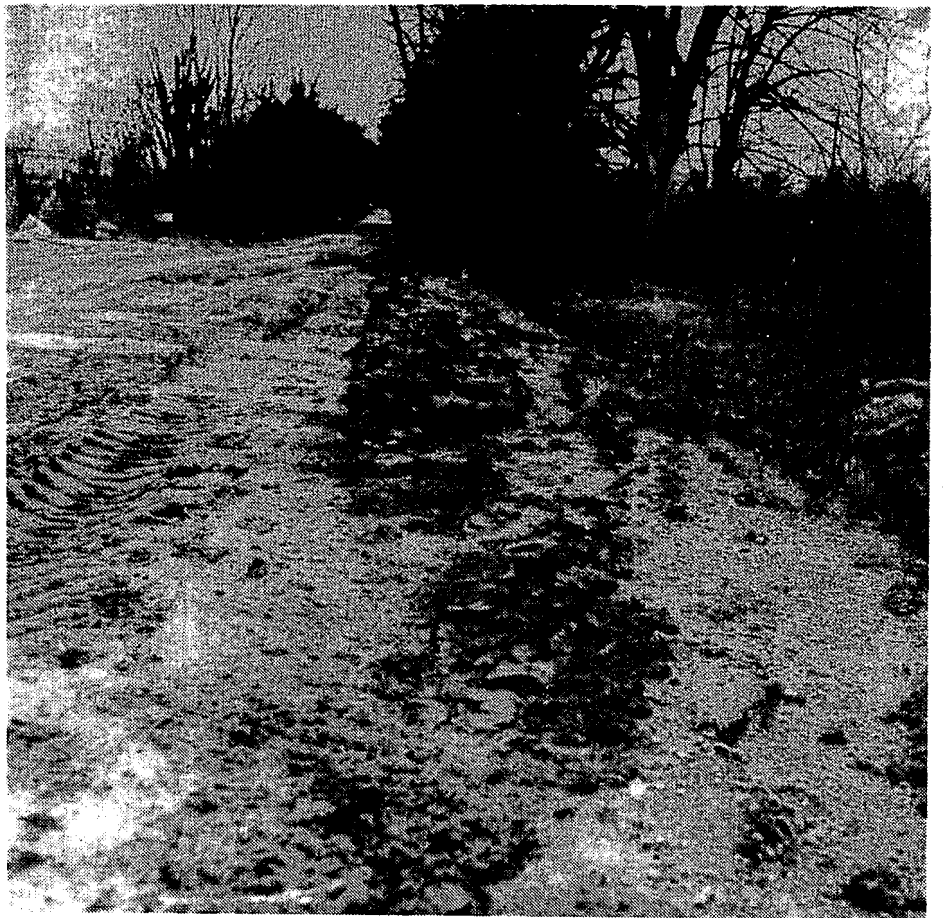
Reese Road was no traveler's paradise as drainage water mucked up the roadbed.
