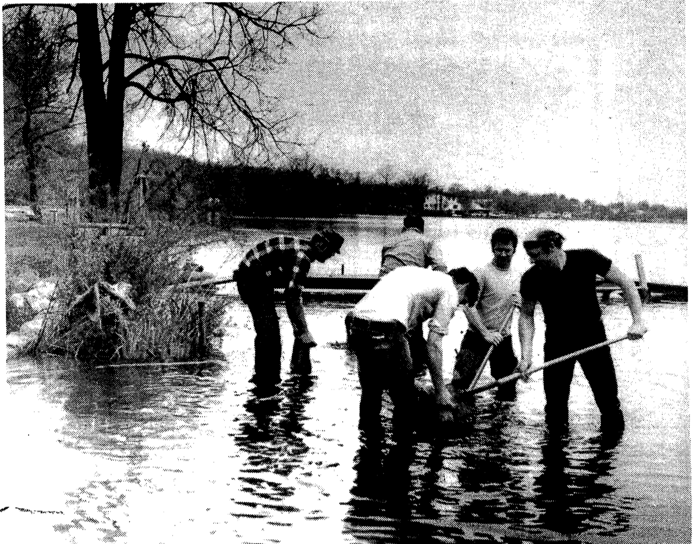
Sunnybeach Country Club Subdivision neighbors worked rapidly to construct a dike at the Walters Lake dam with bags they filled by digging into the lake bottom.
