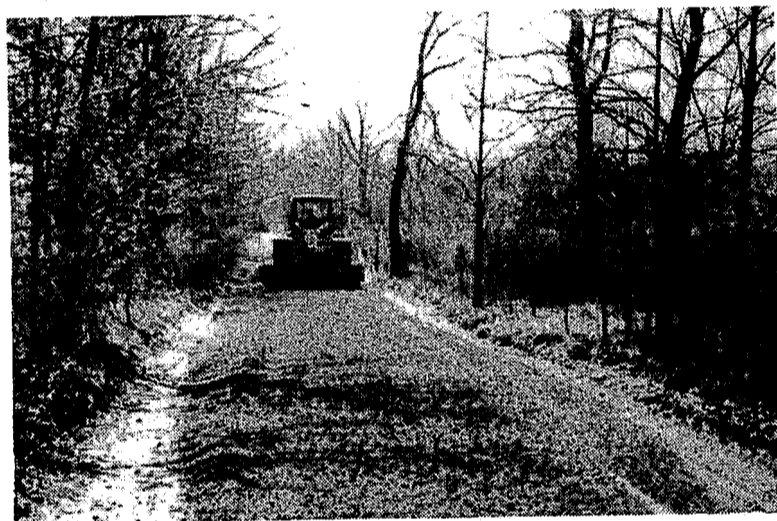
. . . then, during last summer and fall, scenes like the graveling operation shown above became common as the Road Commission rebuilt 437.5 miles of failed gravel roads under special program jointly funded by 18 townships, Board of County Commissioners and Road Commission.
