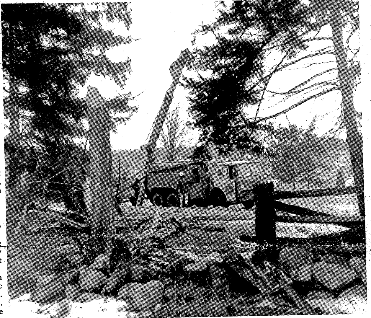
Among the many utility lines which had to be put together by Detroit Edison Company workmen were some on Waterford Hill, torn when a tree was blown over Friday night.
