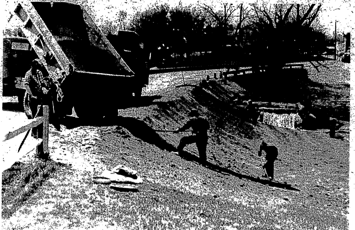
Work began Wednesday on Davisburg Road by the Oakland County Road Commission, and by Monday there were two lanes of traffic once again. The road was washed out by Mill Pond flooding April 18. The Road Commission will have to apply for reimbursement for all the repair work in the county from the storm in a separate request from Springfield's, supervisor Don Rogers said.
