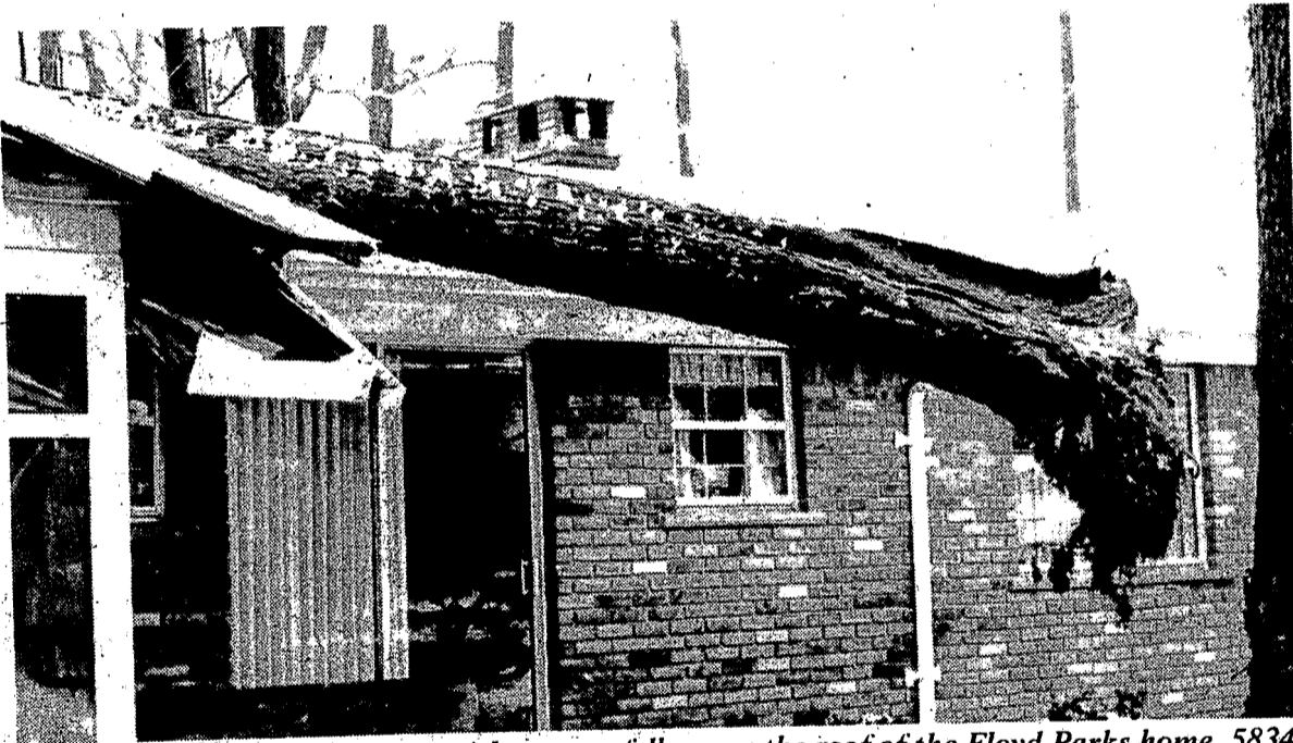
A large tree fell across the roof of the Floyd Parks home, 5834 Kingfisher.
