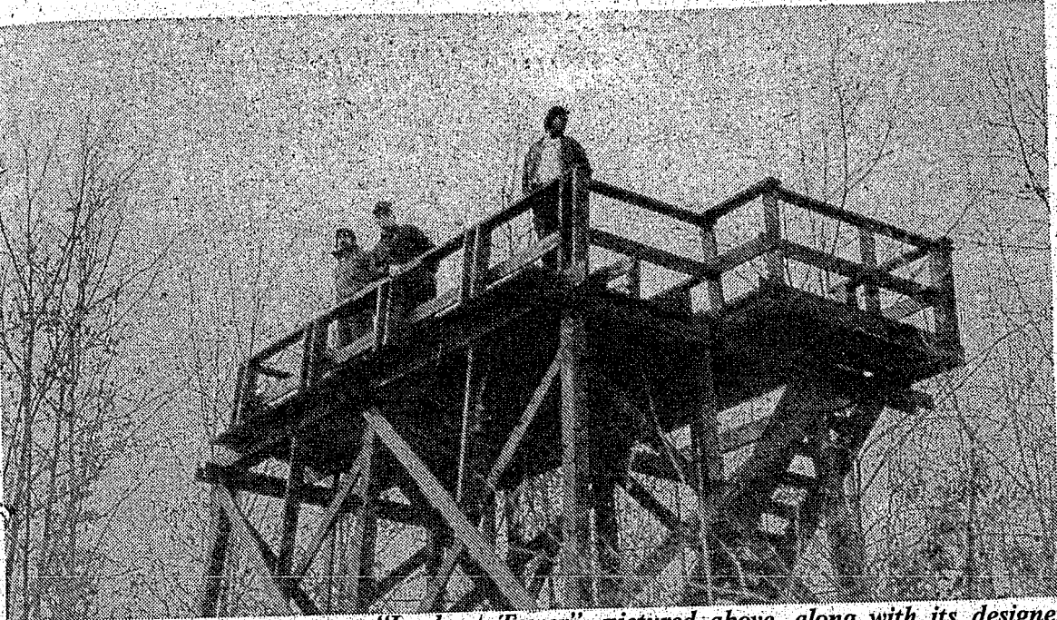
"Lookout Tower", pictured above, along with its designer Johannes Leiting [center], and construction assistants Dave Madrigal [left], and Bill Klosky [right], is the most recent development at Independence-Oaks County Park. The 12' tall structure, situated at an elevation of 1200' on the Rockridge Hiking Trail, provides hikers and cross-country skiers with a panoramic view of Independence-Oaks, Crooked Lake, and most of Eastern Oakland County.
