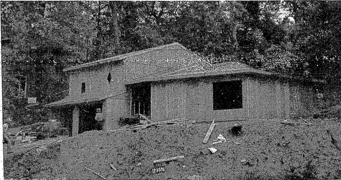
STILL A SHELL. Area Builder Geoffrey Bowman began a home for the Bernard Loague family of Clarkston in the Spring
