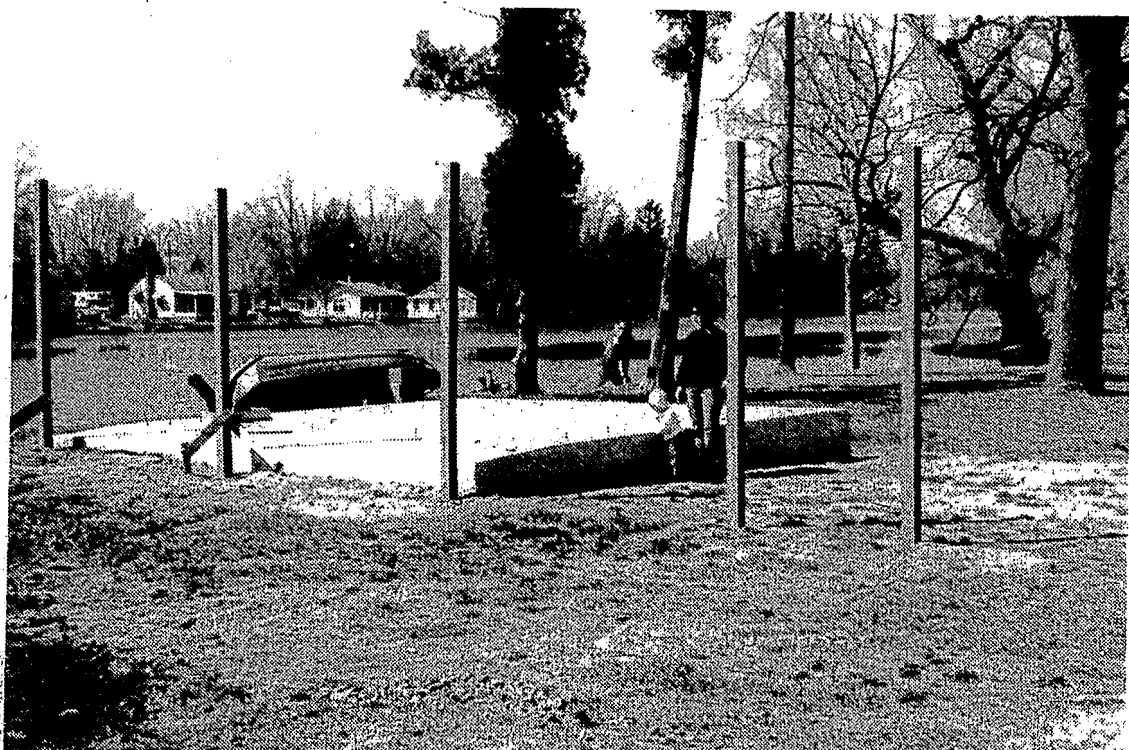
Jennifer Radcliff and daughter Rebecca stand near the slab of cement—an intended foundation for a screen house.
