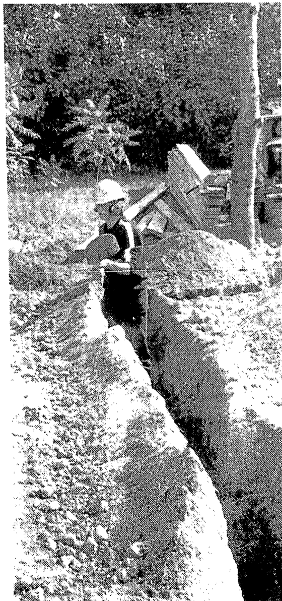
Daryl West, a senior, digs a trench for footings for a concrete driveway.
