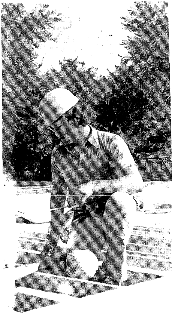
Claus Diemer, a junior, lays out a window opening in a wall which will shortly be lifted into place.
