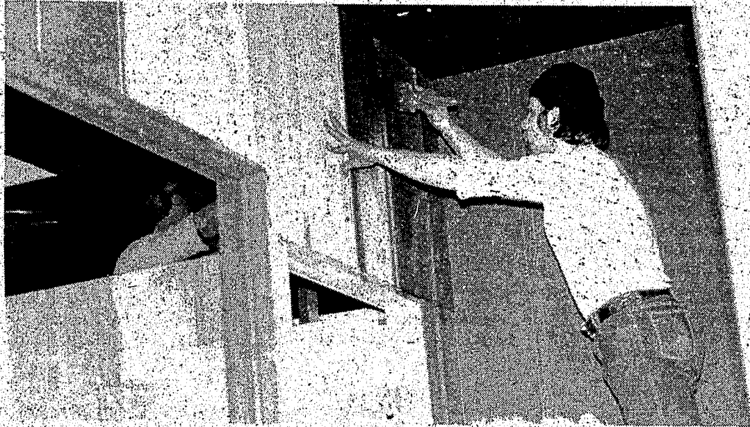
Kelvin Perkins of Waterford Township puts the final varnishing touches on a wall recently built in "Heaven," a youth-oriented bar on Dixie Highway in Drayton Plains. Perkins and "Heaven" owner Joe Puertas constructed the wall to literally divide the bar into two rooms to separate over-21 drinkers from underage patrons.
