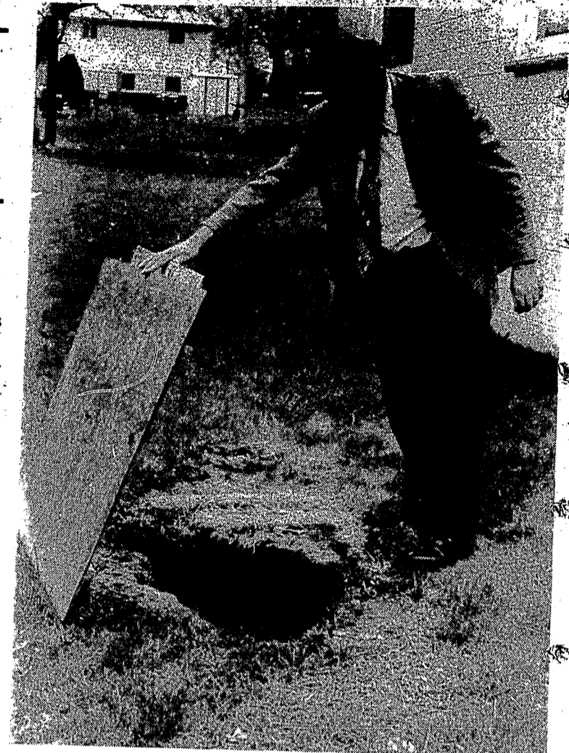
A collapsed portion of the drain results in a gush of water flowing out of this hole in a neighbor's back yard during heavy rain storms, Severance said.
