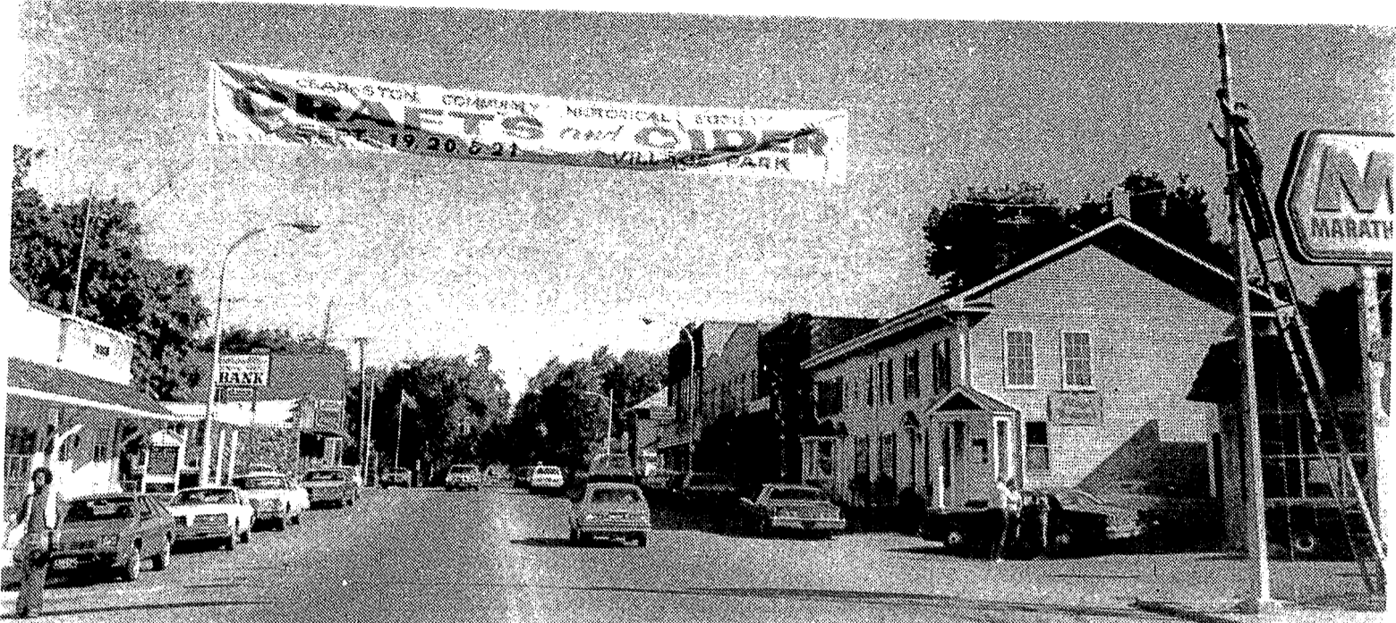
Members of the Michigan Bell construction crew gather to raise high the Crafts and Cider banner over Main Street Clarkston on Friday. The event that features arts and crafts by over 65 artists and craftspersons and food items like honey, cider and doughnuts is to be held Friday, Saturday and Sunday, Sept. 19, 20 and 21 in the Clarkston Village Park on Depot Road. This is the sixth year for the festival that is sponsored by the Clarkston Historical Society.
