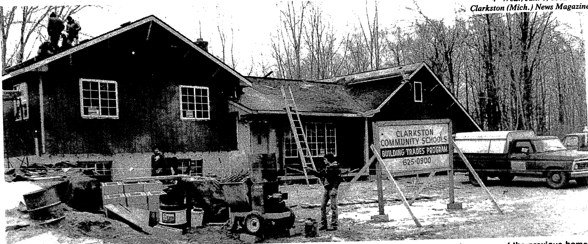
From interior to exterior to the roof, activity abounds at the Clarkston High School building trades house on Goldfinch Lane in Independence Township. This latest house is a little smaller than some of the previous homes built by CHS students.
