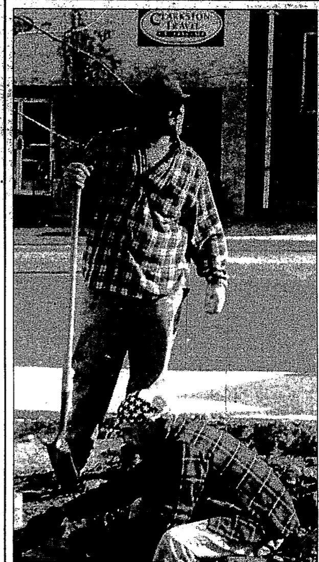
Stars and stripes everywhere -- While our staff was out and about we noticed construction worker Dennis Robinson, not for the fine job on the downtown parking lot, but for his dew-rag. Seems everybody is showing their patriotism these days and we like it. Photo by Jeff Patrus
