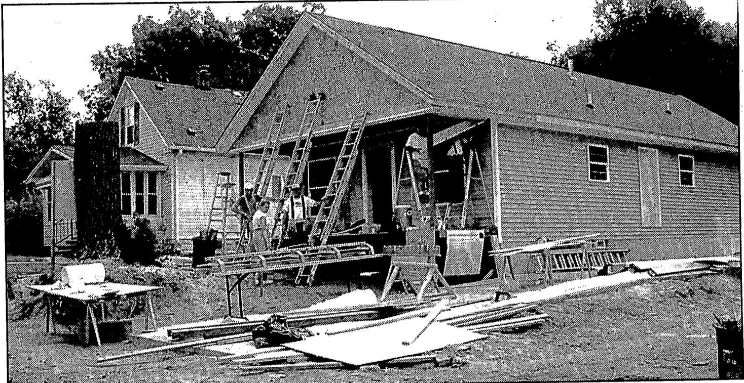
Crew members continue working on the exterior of Onie Morgan's new home as part of Oakland County's Habitat for Humanity "Blitz Build" Aug. 22-28. The Clarkston Christian Coalition helped sponsor the home Morgan moved into and were on site all weeklong to volunteer help. Photos by Alicia Dorset.
