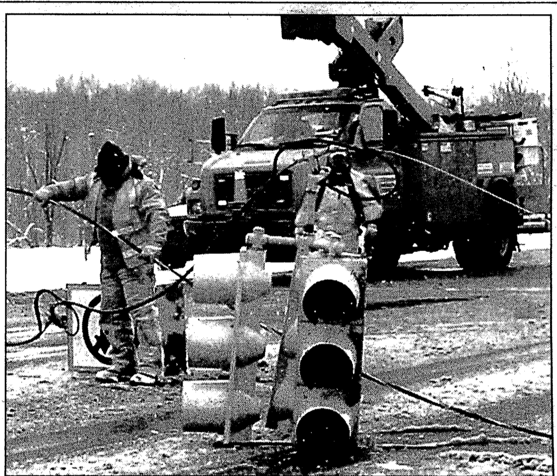
Road Commission for Oakland County employees work to remove traffic signals from M-15 at the northbound exit ramp from I-75 just before 9 a.m. on March 12, after a vehicle ran off the road and snapped one of the support posts. Photo by Don Schelske
