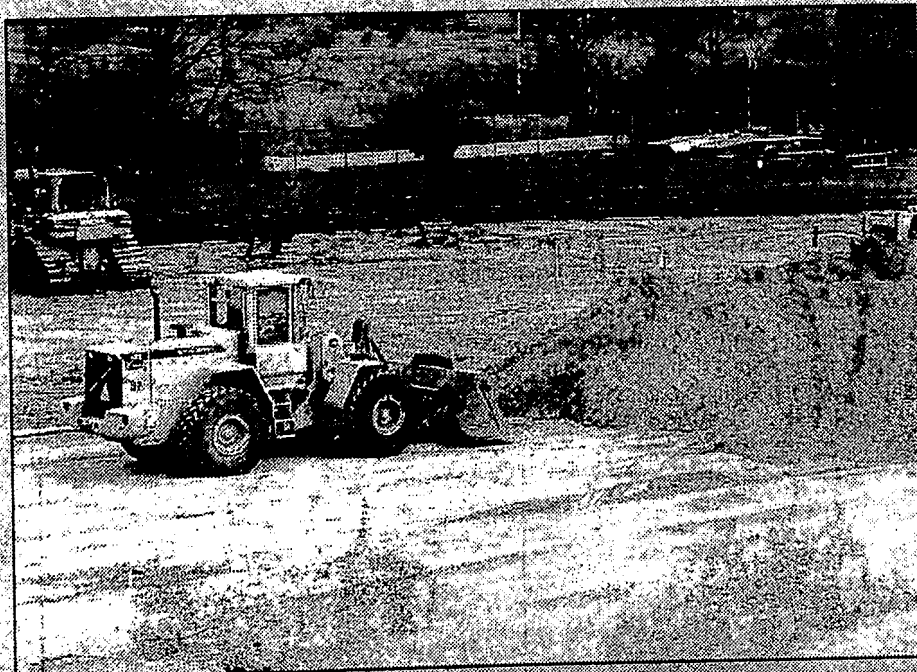
The Clarkston High School stadium has just begun its massive transformation to synthetic turf. On May 3, all natural grass was removed and heavy machinery started to dig out a base. Photo by Noah Purcell
