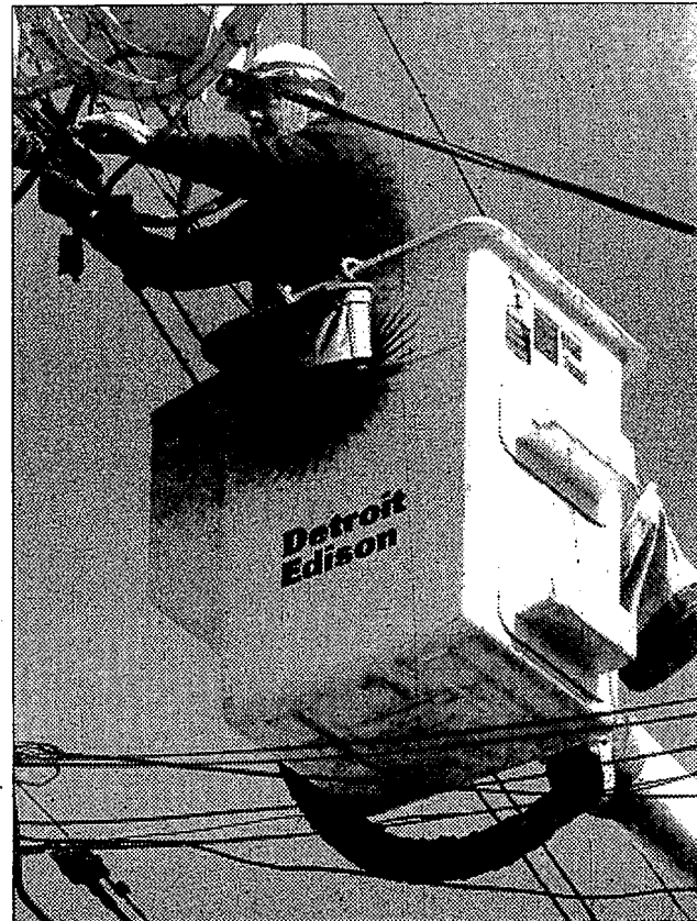
A DTE worker repairs one of three transformers outside the Clarkston News building. Power to the building went down around 5 p.m. May 2, and was not restored until 11:15 a.m. the following day. Photo by Jenny Matteson
