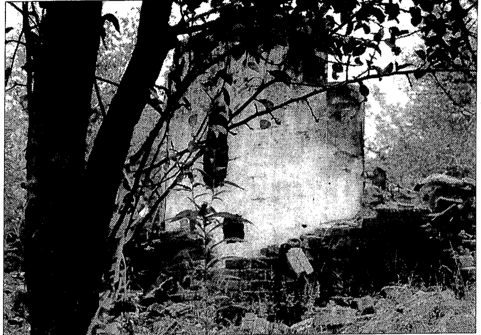
Above, the burnt ruins of a home on Mann Road in Independence Township sits open after the Indep. Twp. Fire Department used the home for practice. Nearby residents have expressed concern over the safety of the property, which contains several open holes, such as the one at left, hidden by thin pieces of wood or tall grass. Photos by Andrew Dupont.
