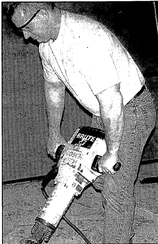
Steve Sitek of Redline Contracting takes a jackhammer to Mesquite Creek's front lobby floor. Photo by Phil Custodio
