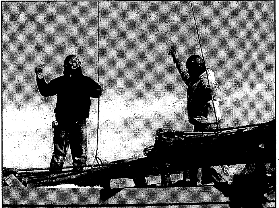
Bill McDonald and Paul Thomas of B&A Steel signal to the crane operator to lift another load. B&A, Connolly Masonry, general contractor Campbell/Manix, and Kieft Engineering are constructing an addition to Chase Plastics on Waldon Road.
