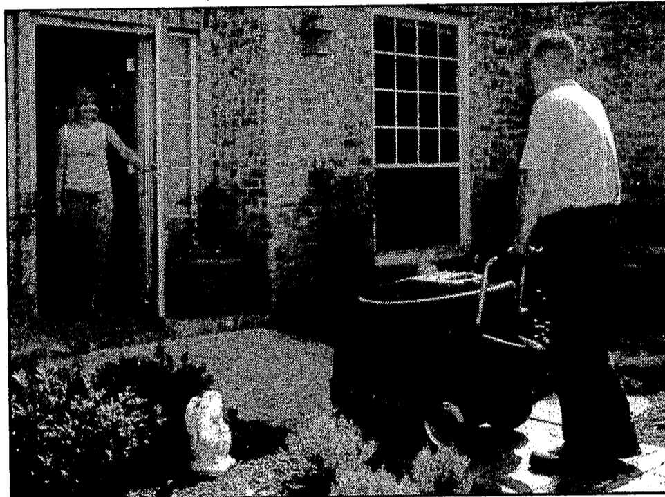
The Home Guy, Inc., uses the Rotobrush Air Duct Cleaning System to clean your home.
