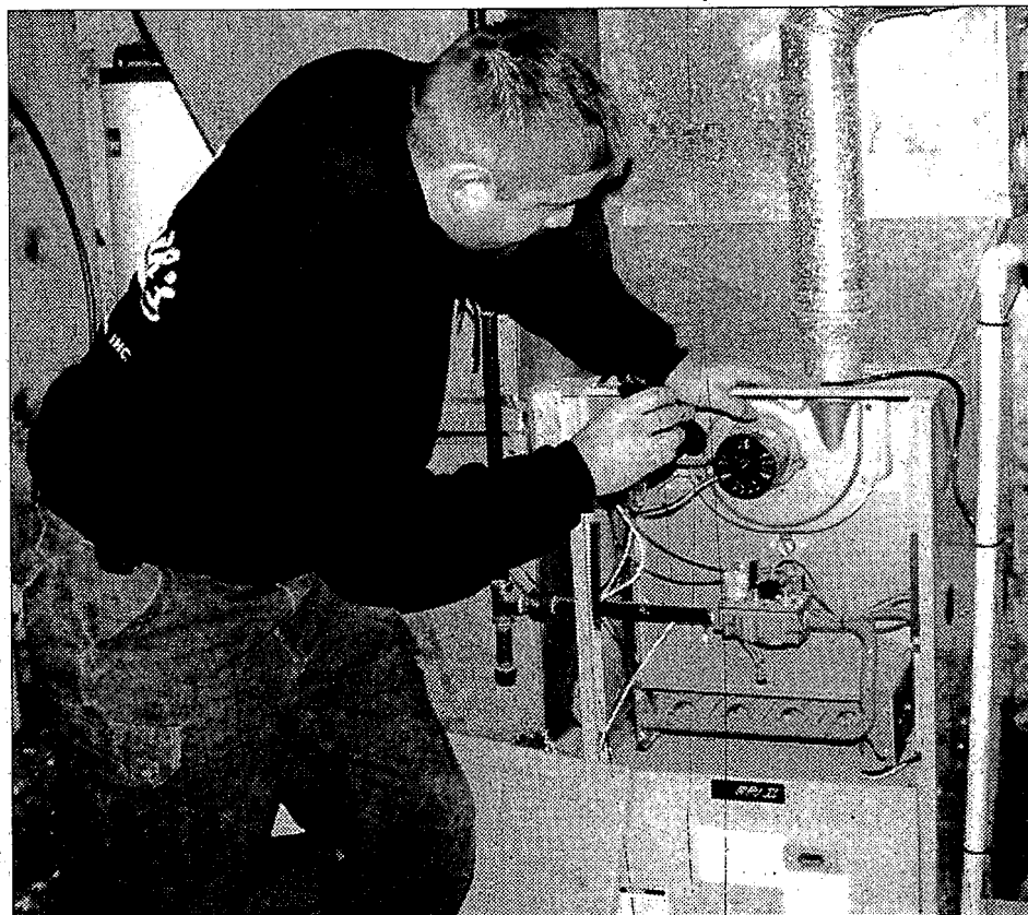
Dan Scribner checks the furnace at 5 S. Main Street. File photo
