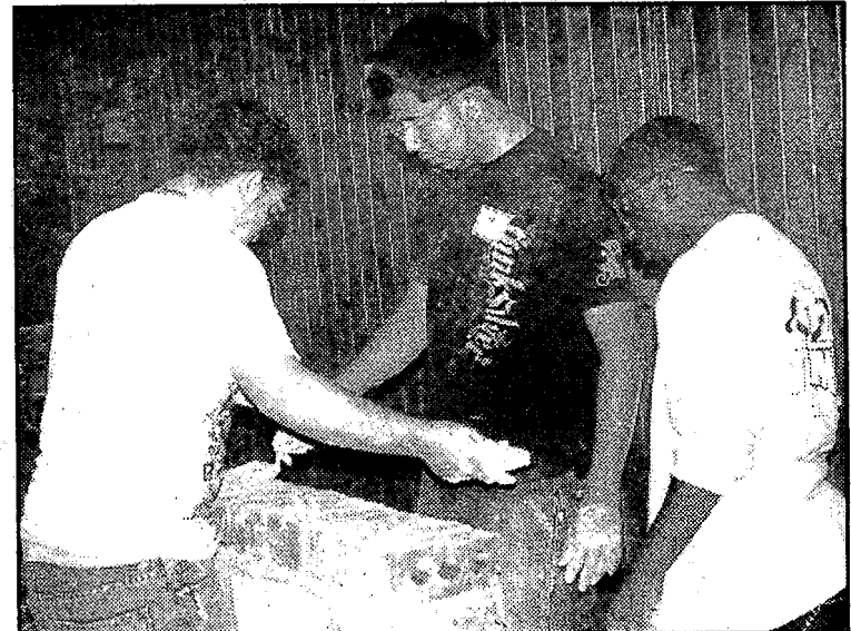
Pablo Salazar Mark Hujan Juan Nawarrete of Ann Arbor build their wall brick by brick.
